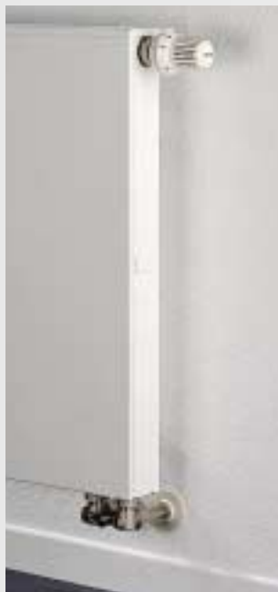
Valve radiator connection from the wall.
