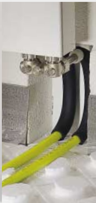
Valve radiator connection from the wall.
